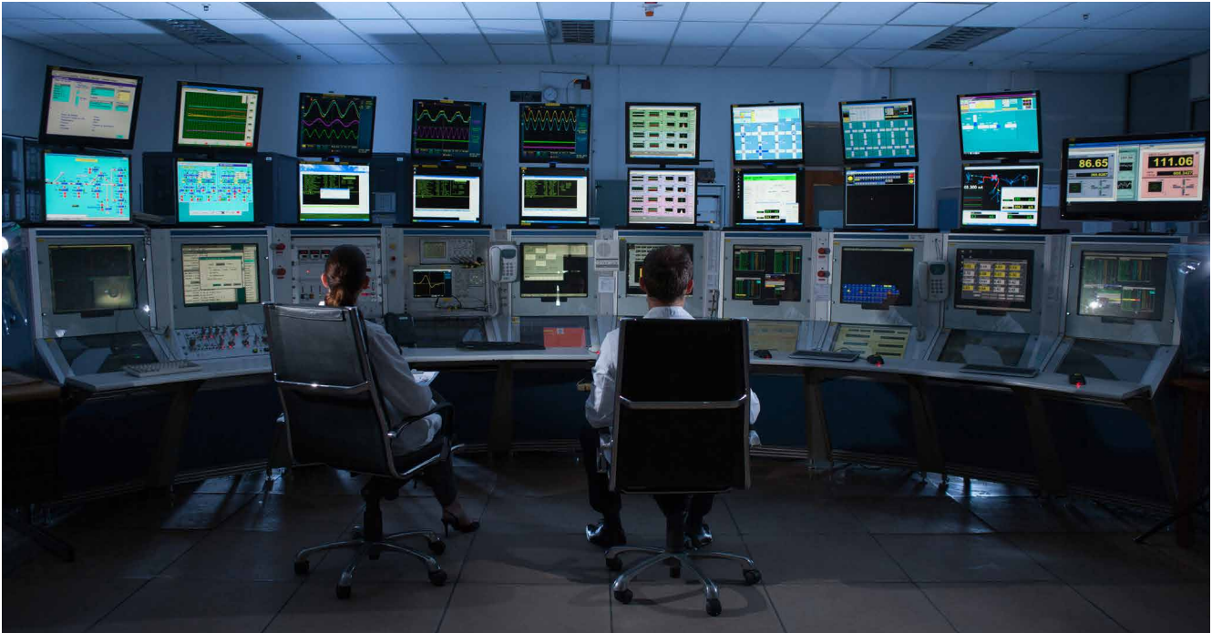
Figure 2. Contemporary control room.
